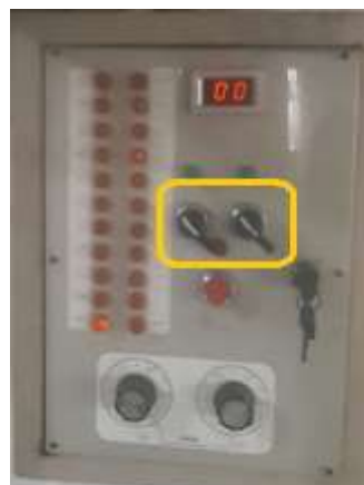
Figure 2. Platform Up and Down Control Panel
