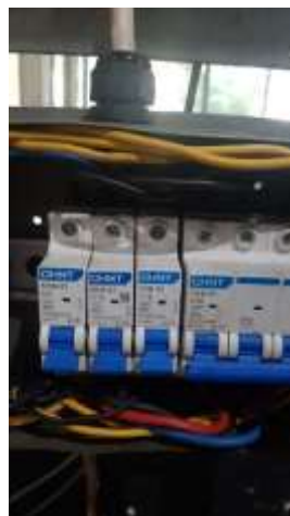
Figure 4. Fuse Renewal with MCB
